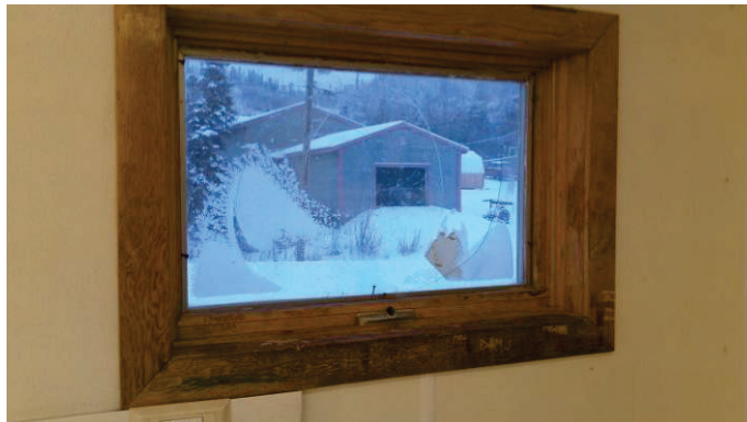
Exterior Window with Broken Pane
